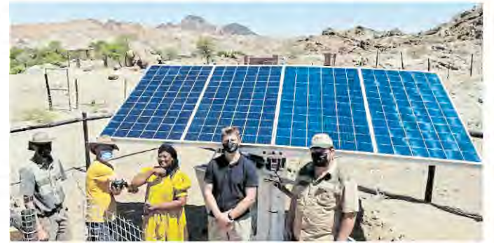
SUN STATION: Elisa Namases and Mandela University students and staff inspect panels used in the solar power installation. Picture: SUPPLIED
