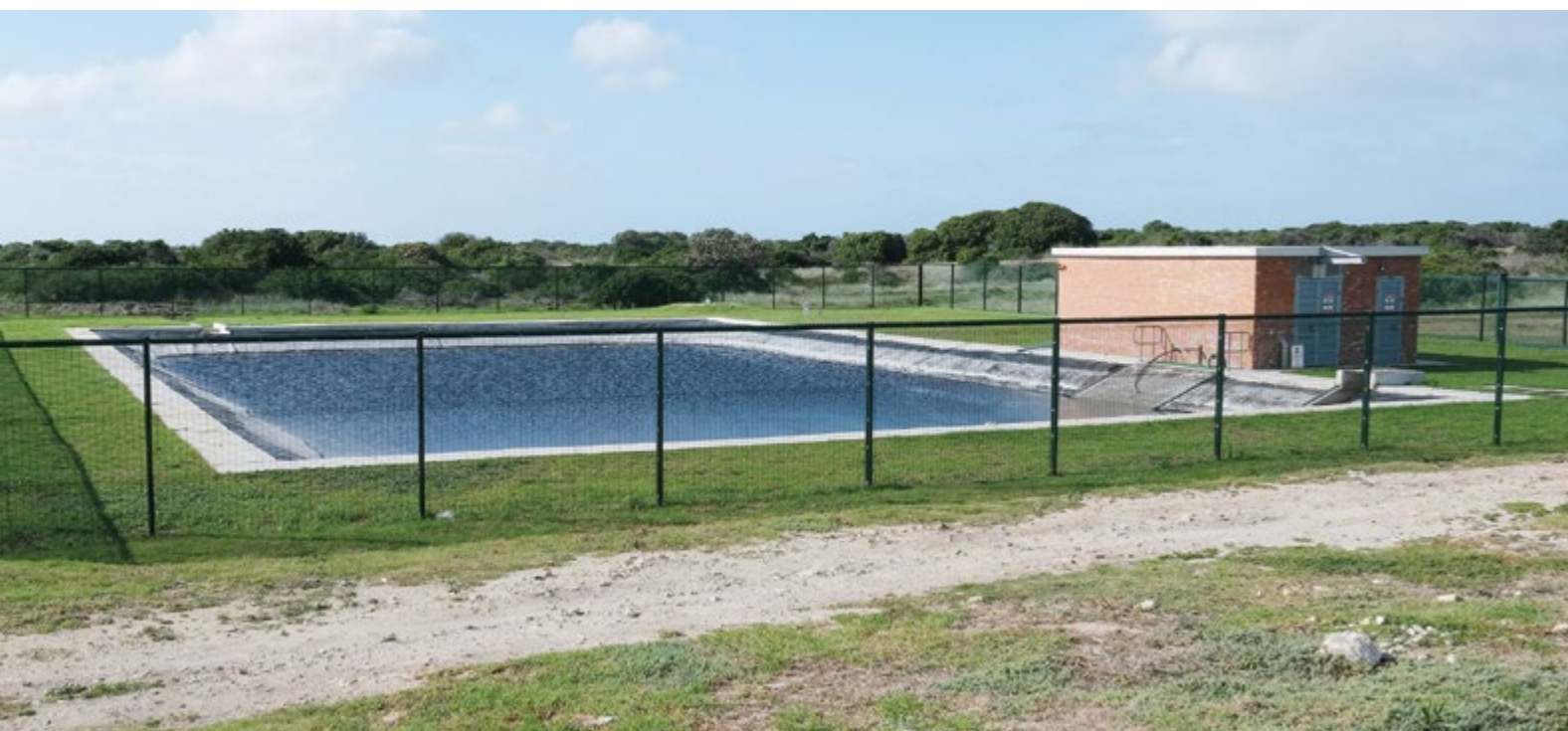
Return effluent retention pond and pump station
