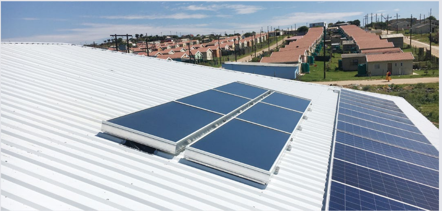
Mandela's new Human Settlement Development qualifications include socially engaged research, such as on this PV solar system in Ndlambe EcoSUN Green Village in Ekuphumleni Township, Kentson on Sea.
