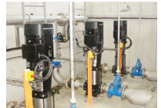
RE water system
