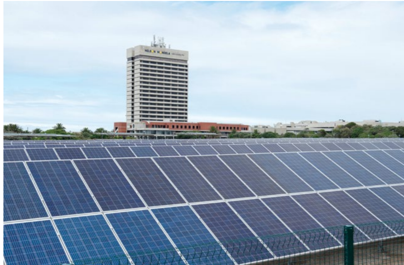
Solar power plant on Nelson Mandela University's Summerstrand Campus
